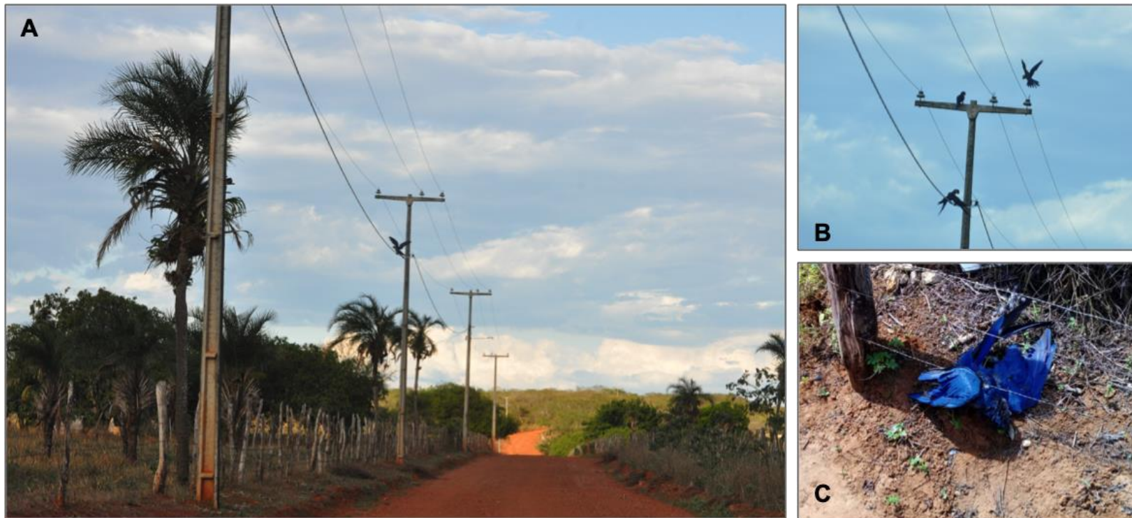
Figure 25 A. Lear's Macaw observed using the power lines during foraging in the Licuri Palm patches. B. Macaws perching in the power lines structures (Photo by Thiago Filadelfo). C. Dead Lear's Macaw found electrocuted under a power line (Photo by Marlene Reis).
